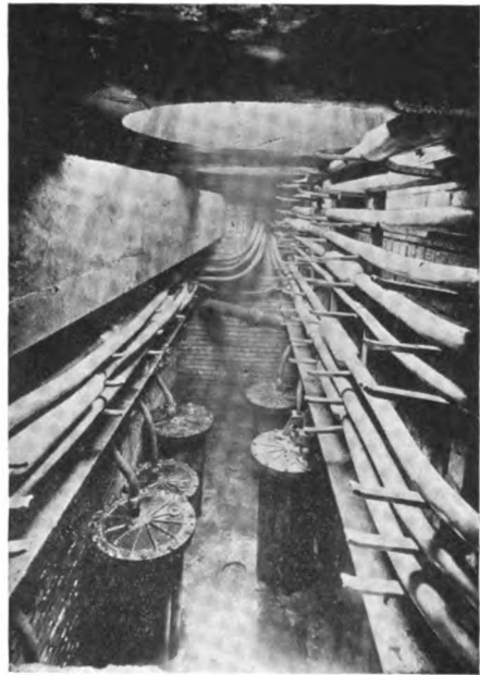
Loading manhole, showing loading coil cases, racking of cables, and at far end, cables entering ducts
