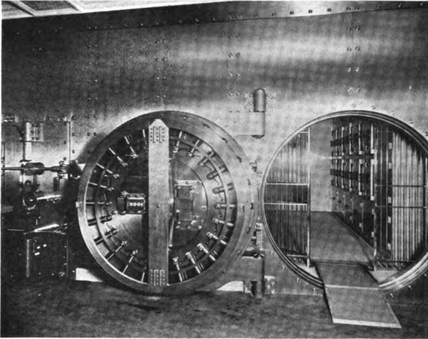
Entrance to the fund vault on the main floor This vault is one of the seven installed by the York Safe and Lock Company
