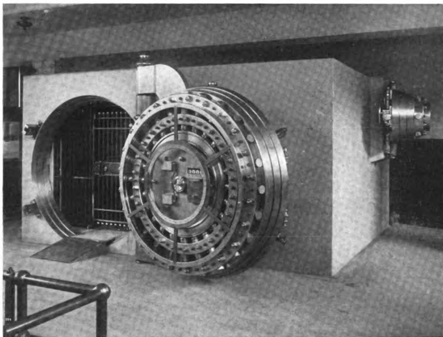
View of Armor Plate Vault made and installed by Bethlehem Steel Company for the E. P. Wilbur Trust Company, South Bethlehem, Pa.
